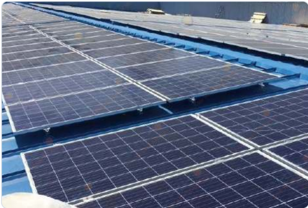
Rooftop PV on metal-tile roof — FRP rail with bolt-on clamps, no
