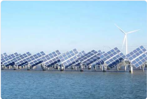
Fishery-PV (aquavoltaic) racking in FRP over brackish ponds
